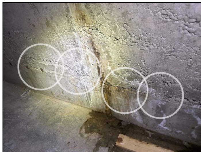
24. Spalling, crumbling or broken material
