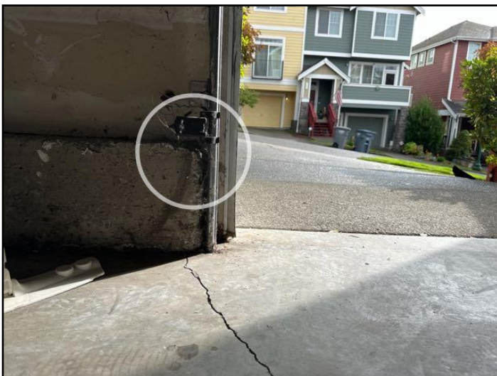
19. Sensors poorly located
