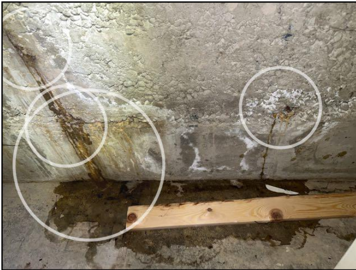
79. Dampness on floor or walls
