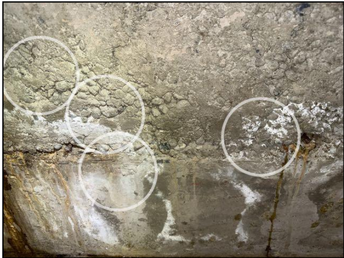
80. Dampness on floor or walls
