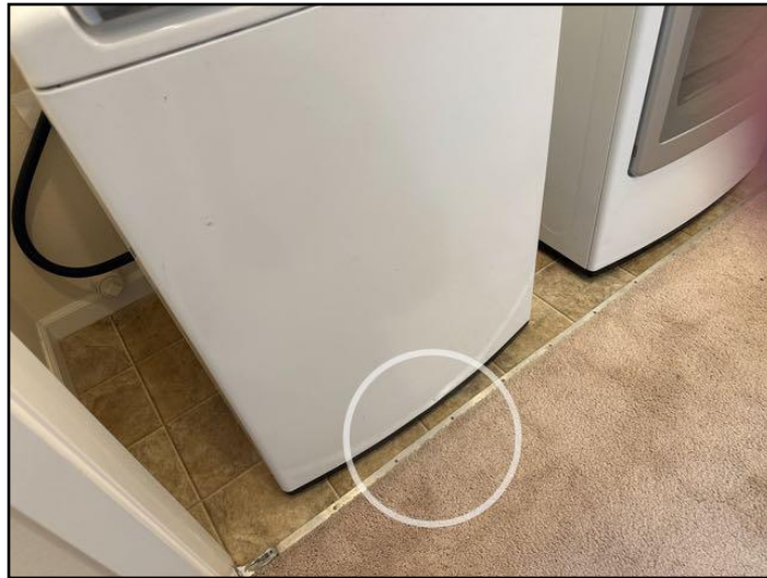
84. Drip pan missing
