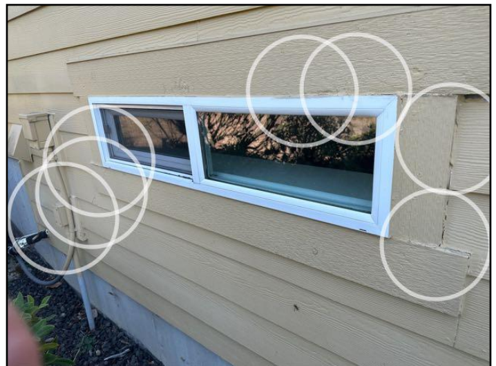
16. Caulking missing or deteriorated
