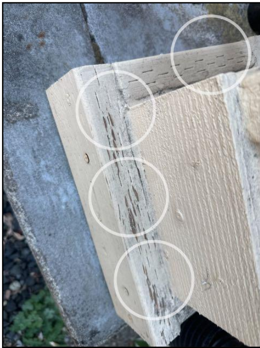
17. Paint or stain needed
