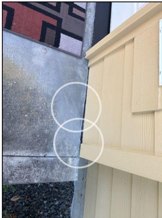
34. Unsealed gap at building
