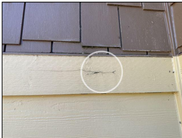
19. Paint or stain needed
