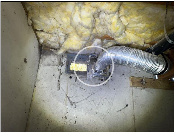
75. Vent disconnected or damaged
