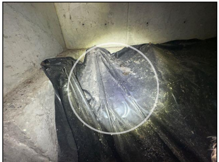
76. Vent disconnected or damaged
