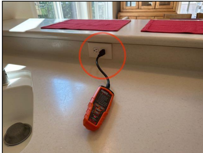
45. Test faulty on GFCI/GFI (Ground Fault..
