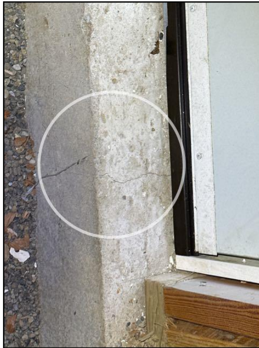
41. Typical minor cracks
